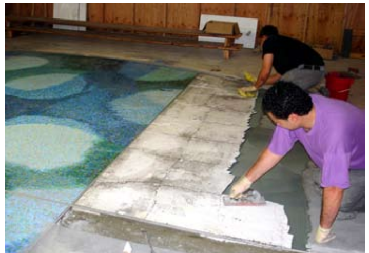
Tile setters carefully tamp individual tile sections into the mortar bed on the Capitol rotunda floor.
